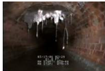
Interfering utility pipe
