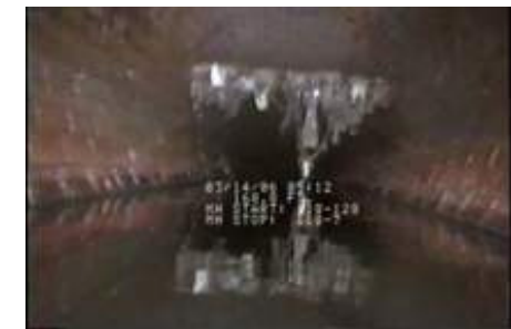
Interfering utility pipe
