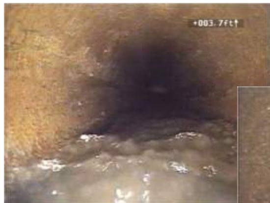
Sag, poor vertical alignment
