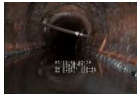
Intrusion, wall mortar loss
