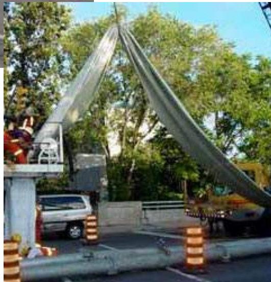
Large diameter Installation: Maintaining pedestrian and vehicular traffic with bypass pumping cross- over points
